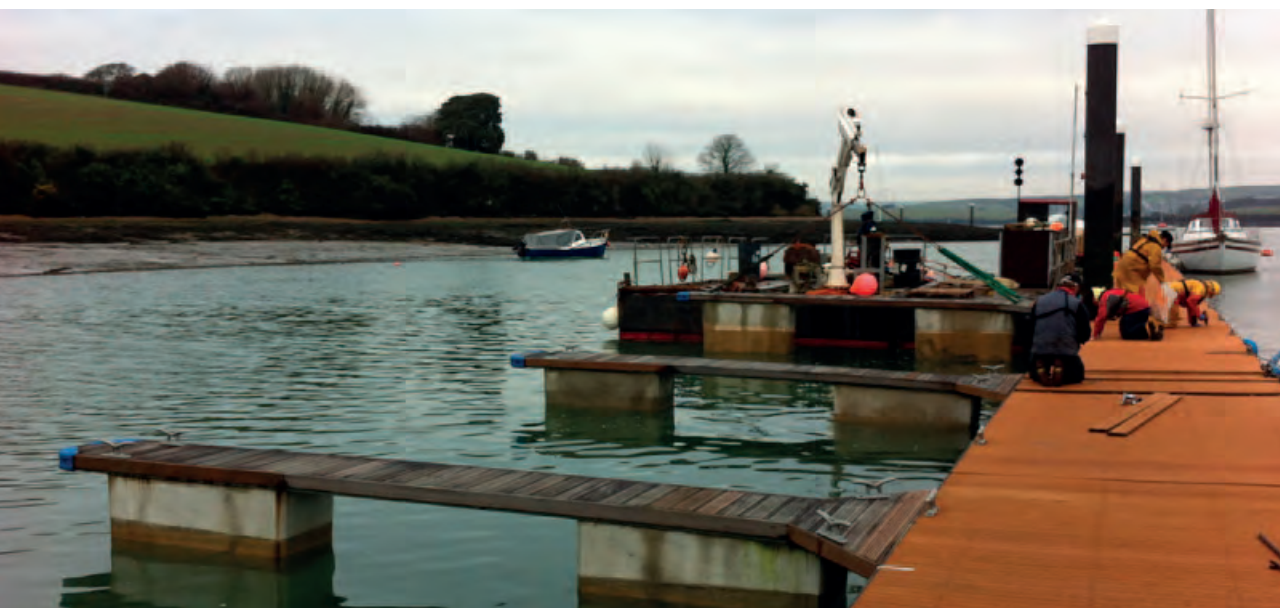
Harbour staff fitting four fingers to B Pontoon in Coad Cove. These fingers will be used for vessels up to 8m LOA
